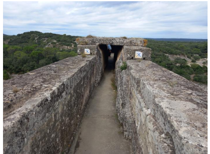
Aqueduct Channel with stone lid. Three centuries of limescale build-up to the side reducing cross section
